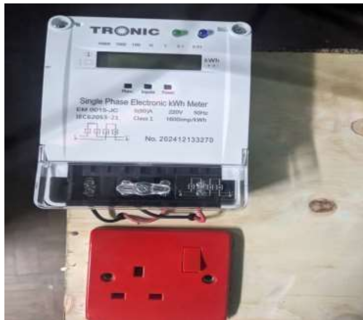
Figure 16: first sub meter
